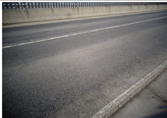
S11 망상균열 (원주방향)
